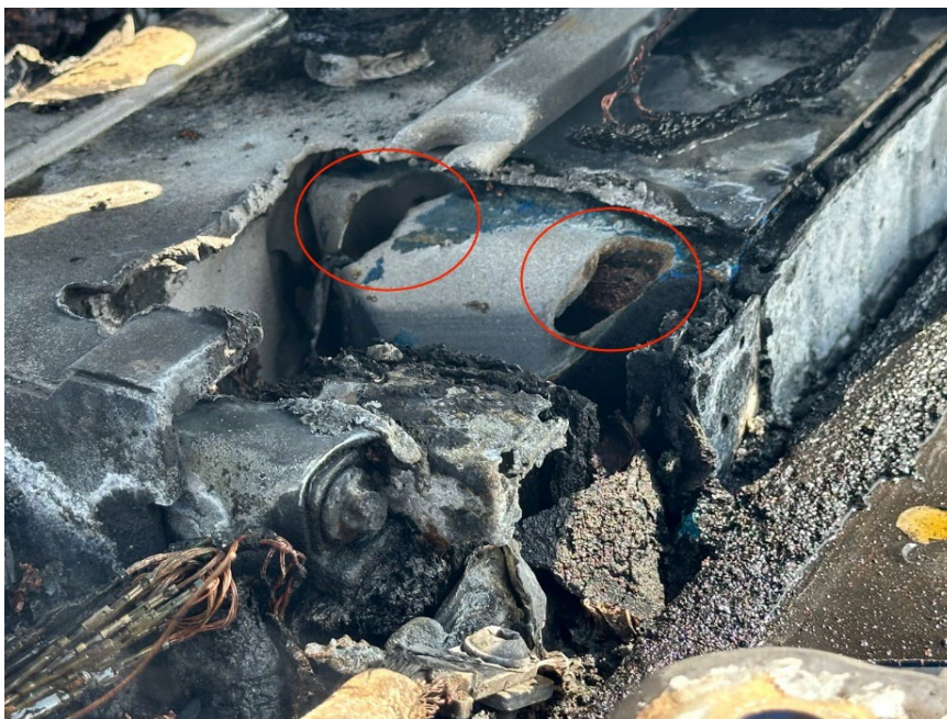
Figure 5.3 Damage or holes after deployment of the UHP extinguishing system
