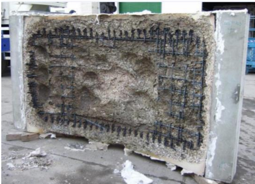
Figure B 1.2 Exposed reinforcement. Photo: MFPA Leipzig GmbH
