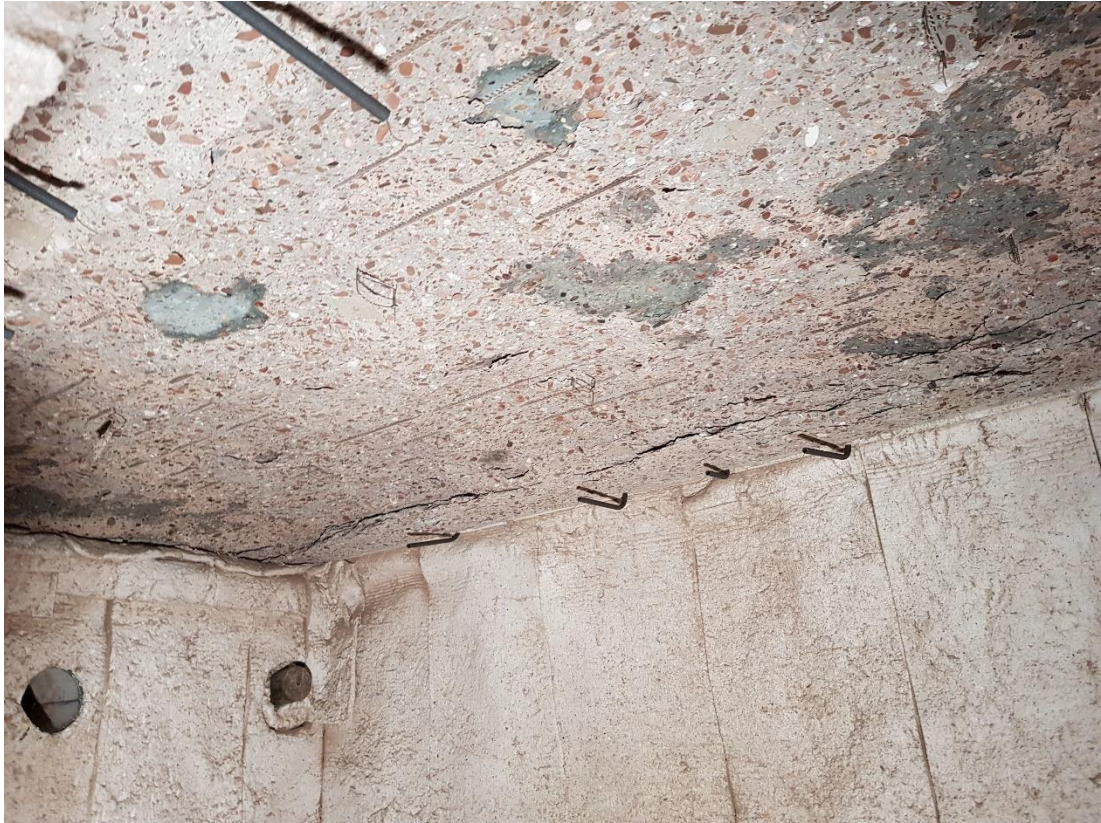
Figure B 1.3 Concrete spalling in the Victory Boogie Woogietunnel (The Hague). Photo: Frank Haring (project organisation Rotterdamsebaan)
