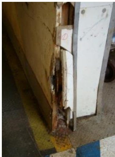
Figure 29 – Damage to Composite Barrier
