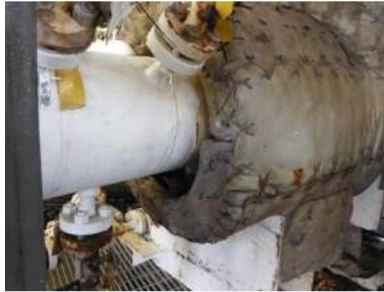
Figure 25 – Poorly Detailed Interface (Component is Missing)
