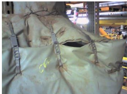
Figure 24 Open joint in jacket-type dry-fit system.
