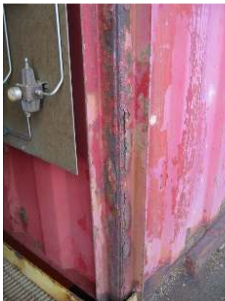
Figure 29 – Corrosion Damage at Fire Barrier Connections
