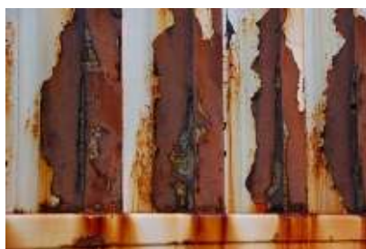
Figure 27 – Corrosion Damage that Breaches Barrier and Exposes Insulation
