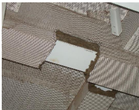
Figure 22 – Mesh retention system (and insulation) not replaced
