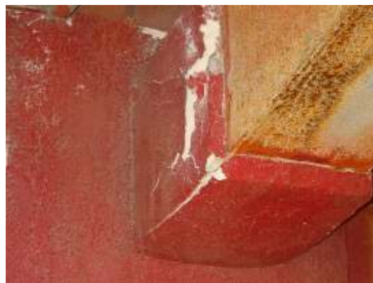
Figure 35- Damaged Cementitious Coating Use to Insulate HVAC Duct
