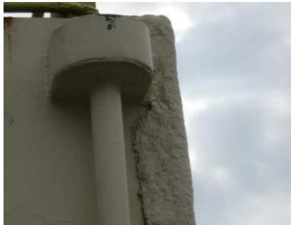
Figure 14 - Poor Termination Detailing of PFP
