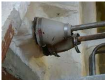
Figure 30 - Incorrectly installed certified gaiter-type penetrations with insulation provided by coating
