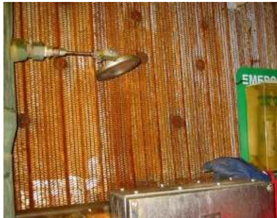
Figure 20 – Corrosion of the Retention System for Man-Made Mineral Fibre (MMMMF)
