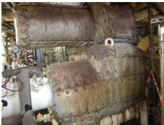
Figure 18 – Contamination to the outer layer of a dry-fit system
