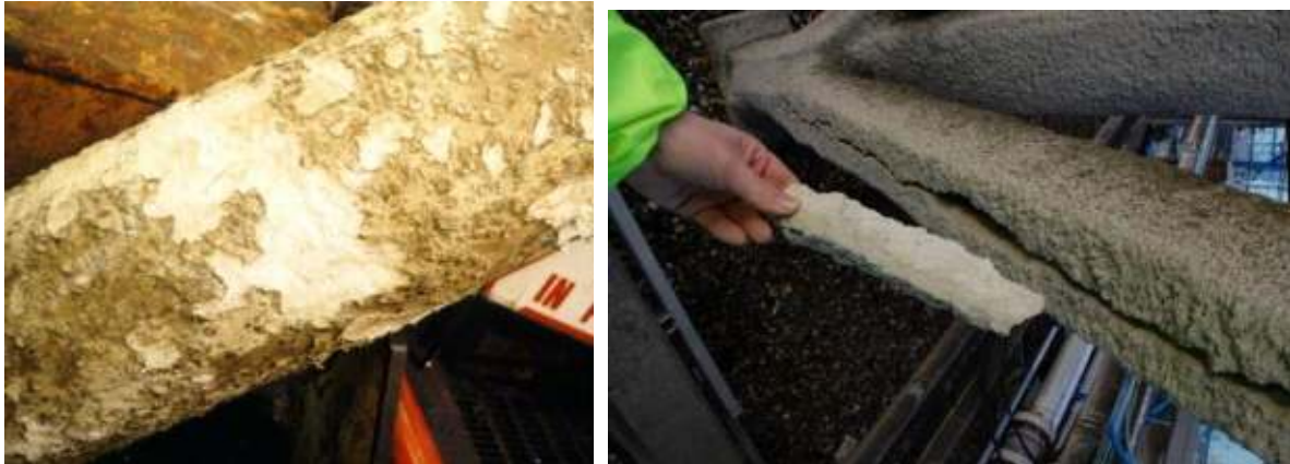
Figure 10 – Examples of Damaged LWC PFP Photographs courtesy MMI Engineering Ltd
