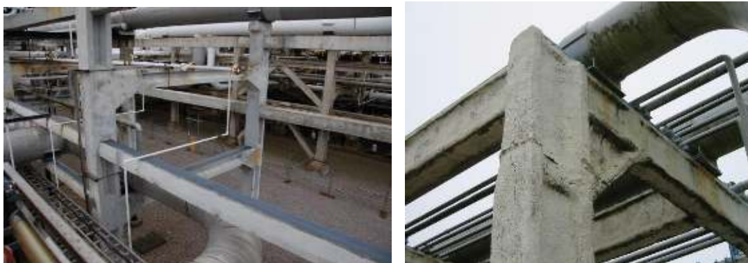
Figure 43 – Examples of unprotected top flanges on beams
