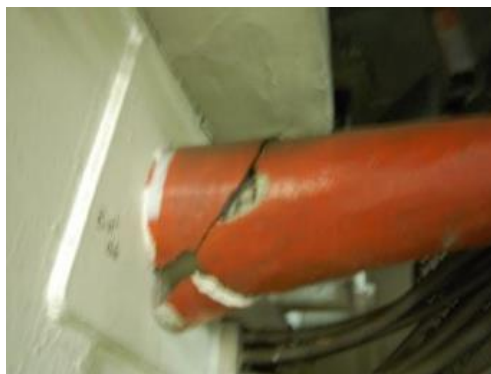
Figure 32 - Damage to Penetration made with LWC material
