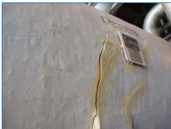
Figure 13 – Cracking of Epoxy PFP due to Thermal Expansion
