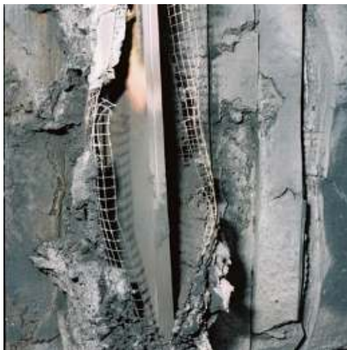
Figure 39 – Reinforcing mesh termination failure
