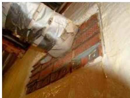
Figure 33 - Cable transits with poor insulation detail to protect cables (Insulation on barrier is in place)
