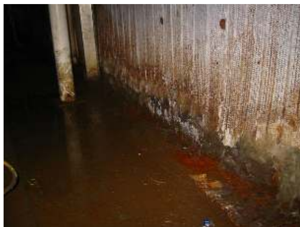
Figure 19 Severe waterlogging damage to retention system of MMMF insulation. Photograph courtesy of MMI Engineering
