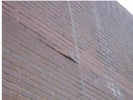
Figure 28 – Breaches in a Brickwork Barrier that Must be Smoke and Gas Tight
