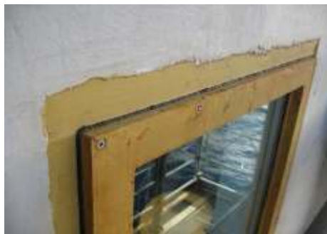
Figure 34 - Missing insulation around fire-rated window
