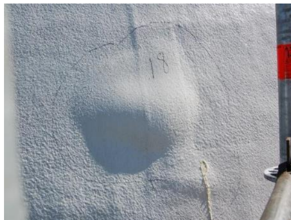
Figure 15 – Blistering of Epoxy PFP Materials
