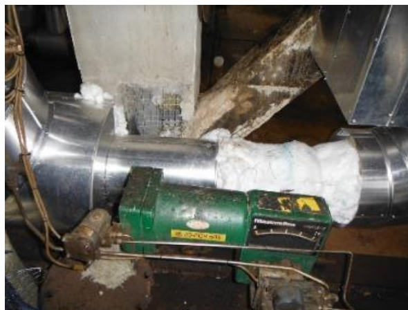
Figure 26 Cladding removed and not replaced.
