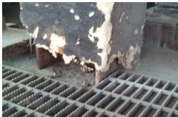
Figure 47 - Damage to Coatings due to Water Uptake
