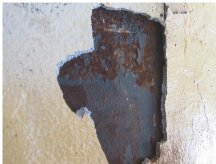
Figure 11 – Disbonded Epoxy PFP
