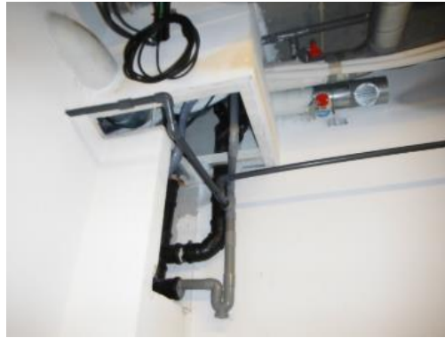
Figure 31 - Penetration not fully sealed
