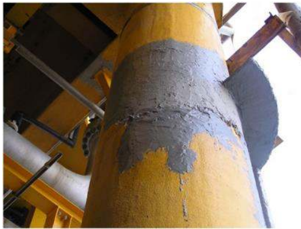
Figure 50 – Badly Made Repair of an Epoxy Intumescent PFP system
