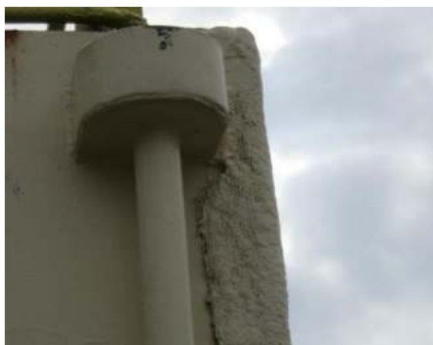
Figure 40 – Badly detailed PFP termination
