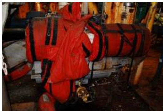
Figure 21 - Incorrectly installed jacket-type dry-fit system (straps are installation aids) Photograph courtesy of MMI Engineering
